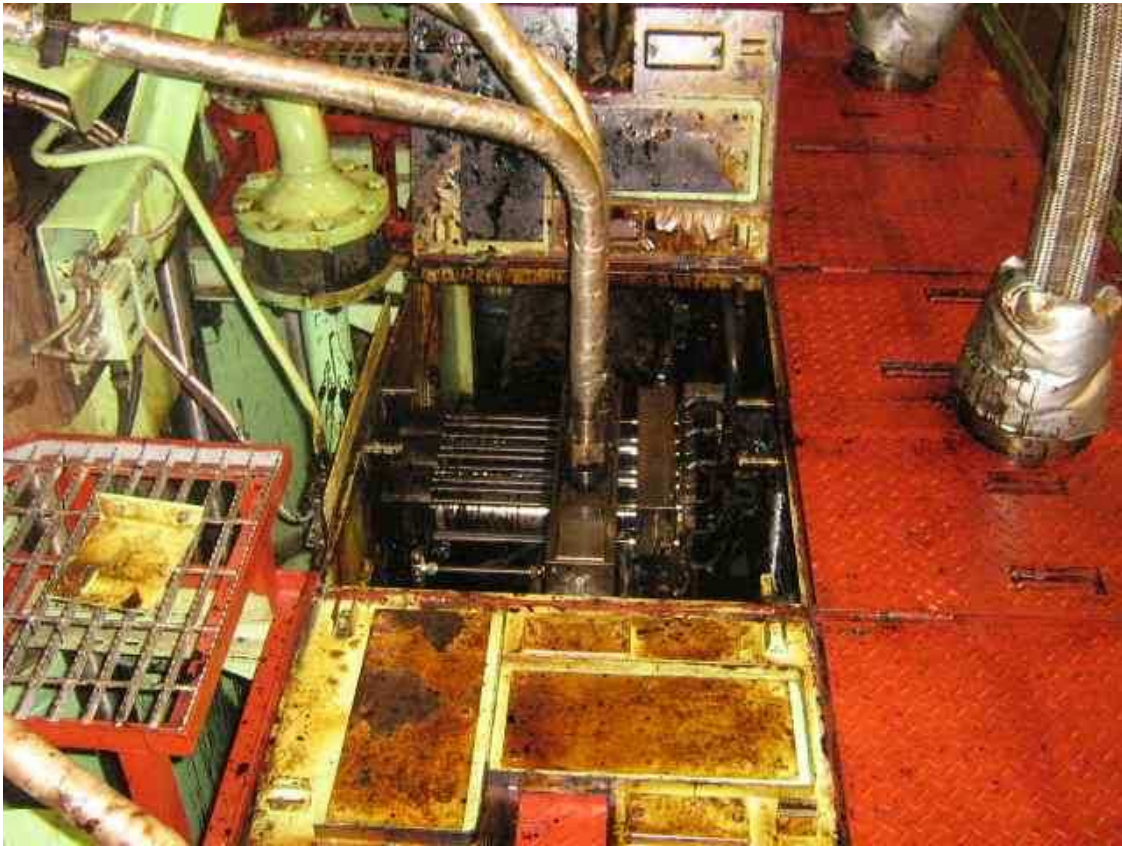
The ICU situated on the fuel oil rail
