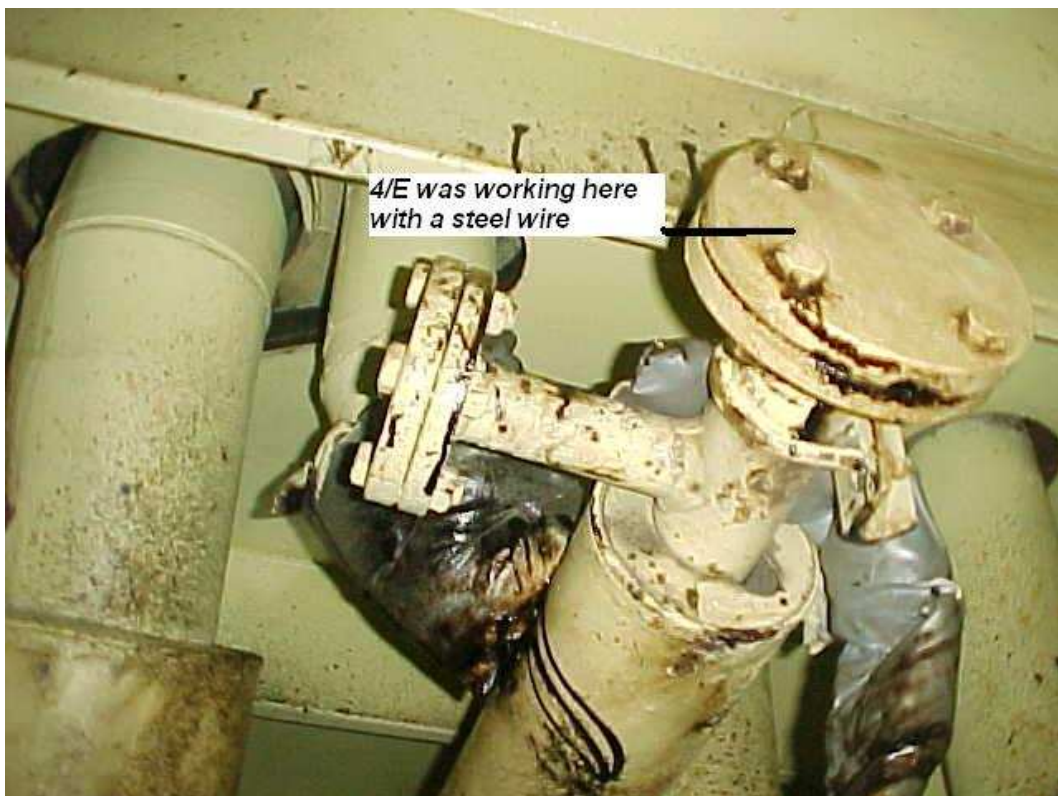
Photo: chief engineer, m/v SORØ MÆRSK
